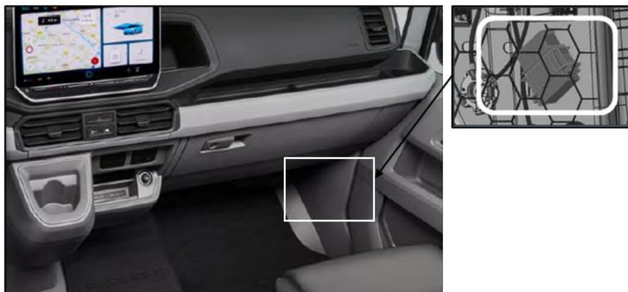
Terminal strip (IS1) behind A-pillar trim, at the bottom
